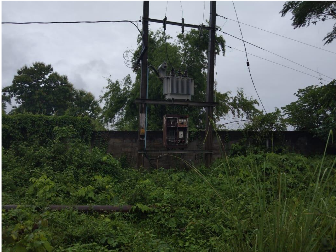
Figure 5. proposed electricity control box and spare part to replace
